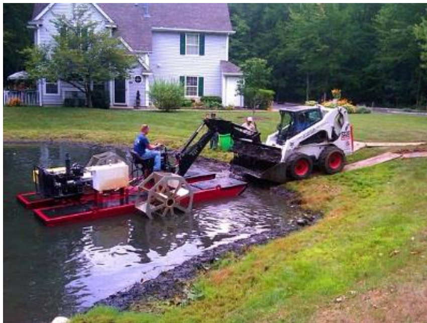
Figure 9. Hydro-rake loading debris right into a tractor's loader bucket. (Aquatic Technologies Inc., 2015)
