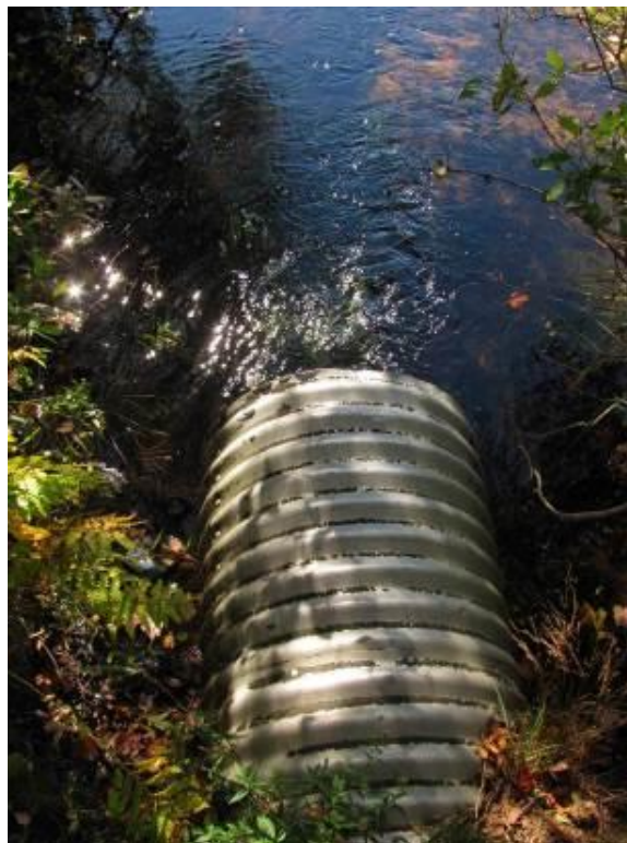
Figure 35. Large metal pipe running underneath paved road into Lake Elizabeth. Photo credit: Danielle Desmarais
