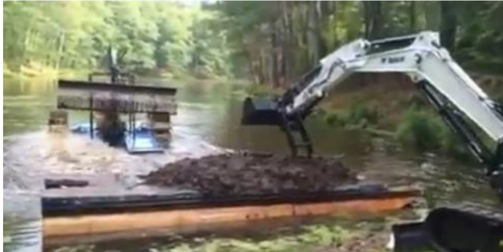
Figure 10. Hydro-rake loading debris onto a floating barge, collected by a loader bucket and placed into a dump truck bed for transport (Tom Largy, 2015).
