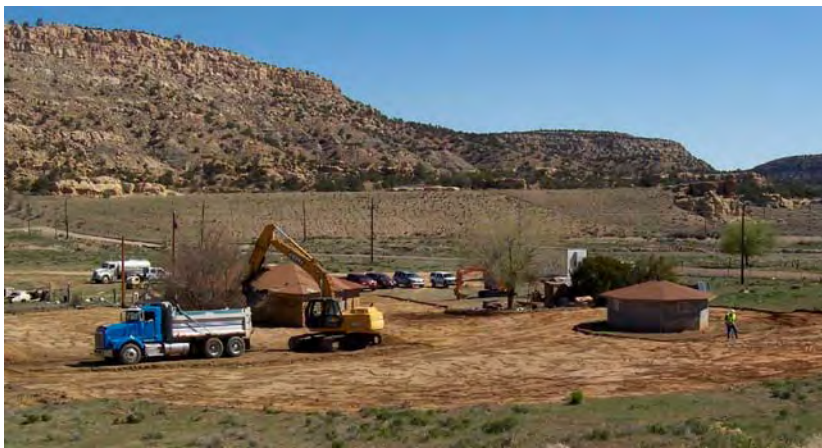
Figure VII.3. Radium-contaminated soils are excavated from around these homes on Red Water Pond Road in May 2007. The reclaimed Church Rock I Mine site forms the ledge in the middle background.
